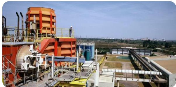
SOLAMAT-MEREX for hazardous industrial waste incineration (France)
